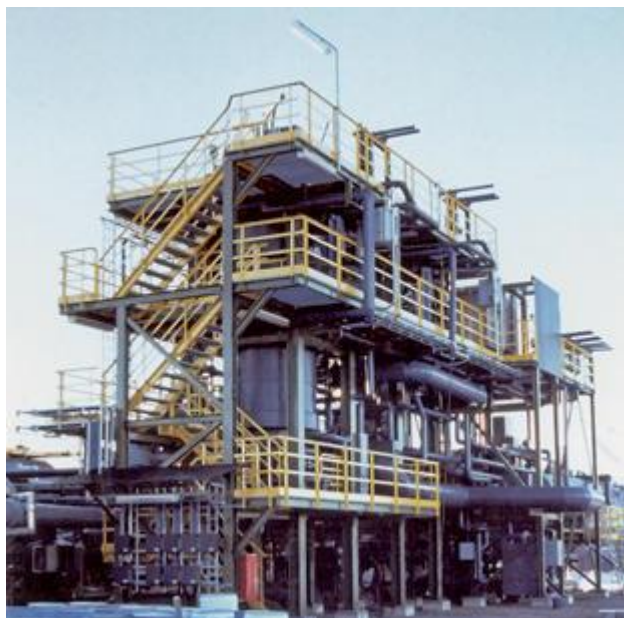
Figure 13-1: Typical Solvent Recovery Plant 1
